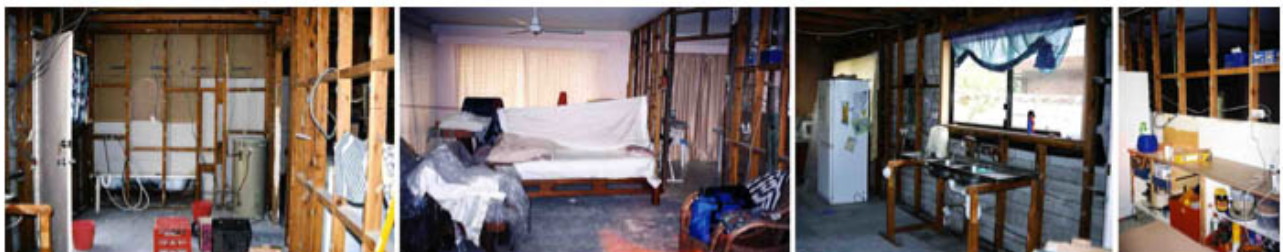
Figure 5 Living in a building site brings daily renegotiation in habitual ways of living. House at Broadbeach Waters, Queensland. Photo: Nicola D Smith 2000.
