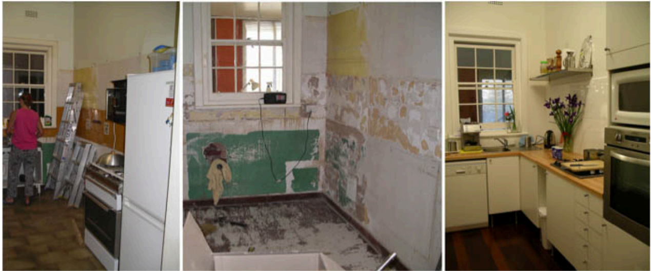
Figure 6 Do the changes we desire - really change our world? Images recording progress of kitchen renovation in Perth. Photo: Nicola D Smith 2005.
